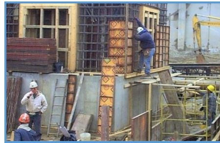
A contractor works without fall protection.
